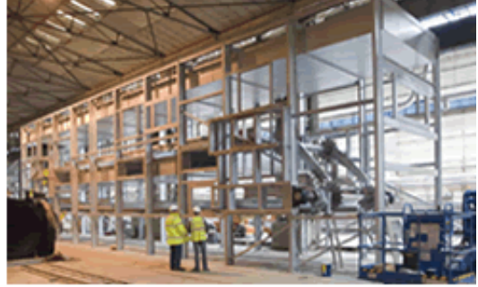
A CDS R-02 Dryer in the pre-build stage
