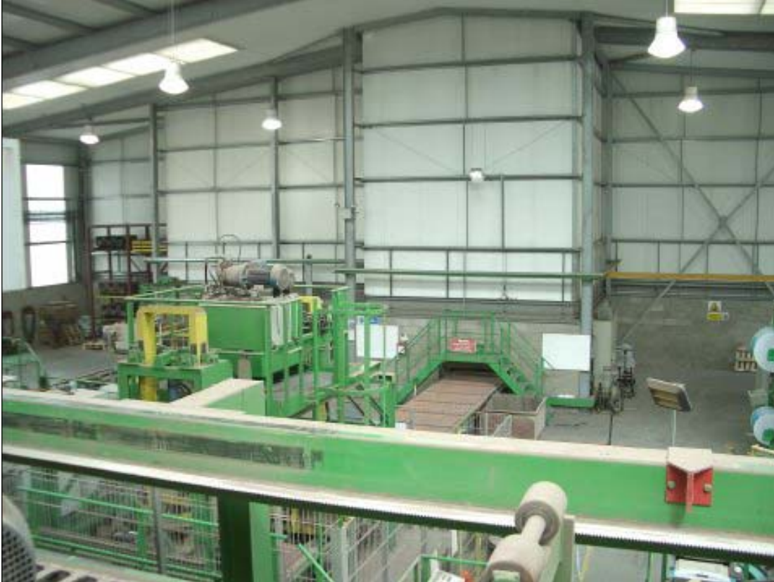
To achieve higher curing efficiency, the chamber, finger car, elevator and, lowerator are totally enclosed within an insulated curing chamber. This photograph shows the insulated cladding panels that form the front wall of the curing chamber.
