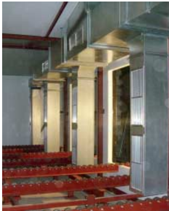
Fig. 3 Internal view showing the hot air supply ducting and the roller conveyor for the handling system.
