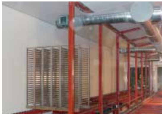
Fig. 2 Internal view showing an empty stillage, internal roller conveyor, support steelwork, angled roof construction and high level exhaust ducting.
