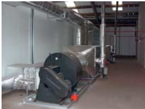
Fig. 7 Rear view of the oil fired air handling unit and insulated supply/recirculation ducting.
