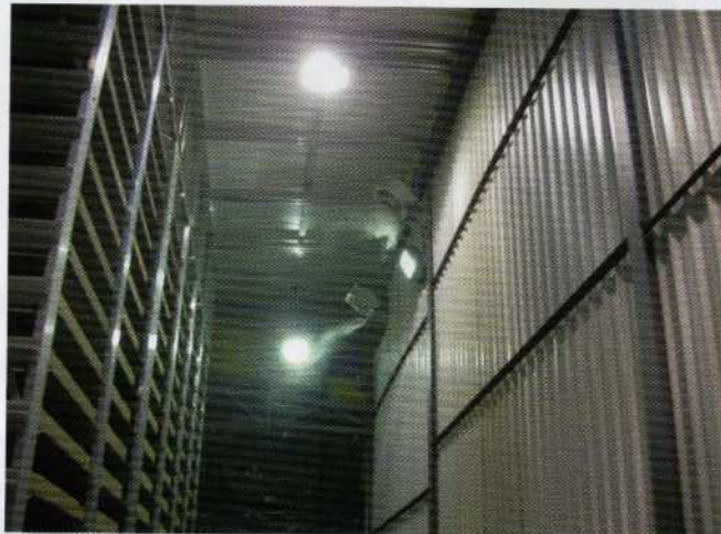
The CDS Envirocure System installed at Tudorstone uses independent control of temperature and humidity allowing the ideal conditions for the process to be set
